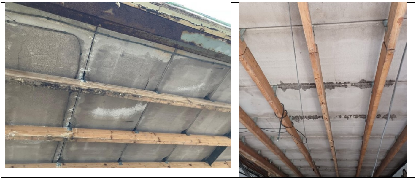
Figure 20 - External Walkway - Unsupported modified planks, surface cracking and efflorescence from moisture
