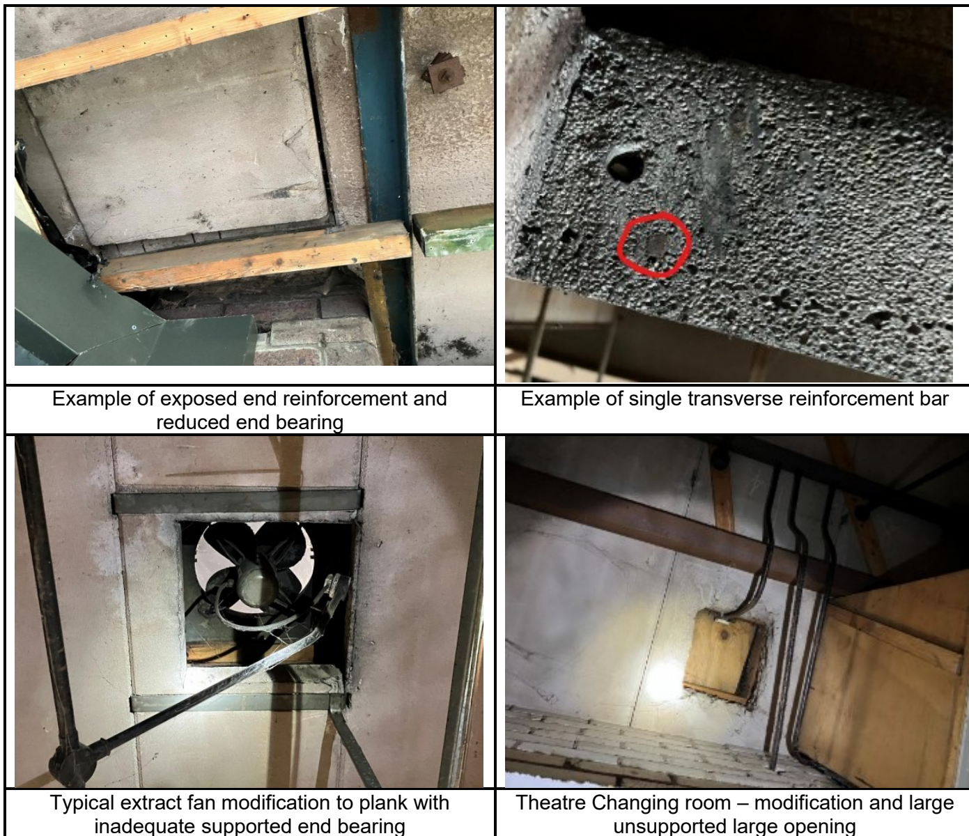
Figure 16 - Examples of modification and penetrations to planks. Source Thomas Consulting (2023).
