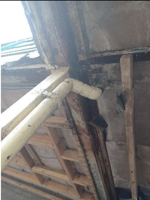
Covered internal walkway RAAC plank penetration, timber beam support and corrosion to steel work beam. Evidence of moisture ingress.
