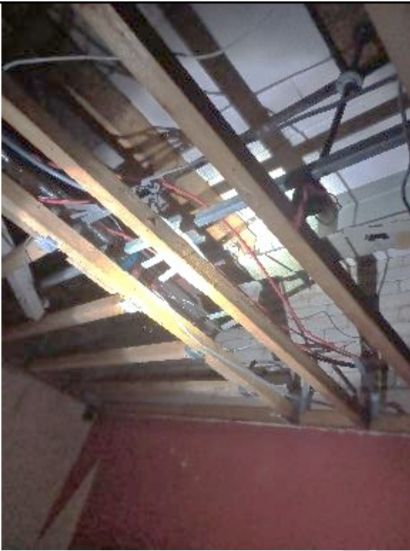
Above suspended ceiling to Social bar area - services
