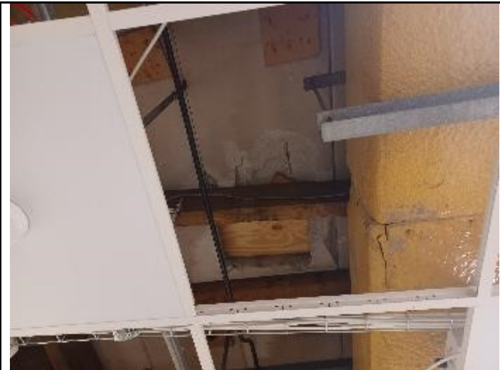
Cut opening to RAAC Plan and damage to concrete exposing reinforcement bar
