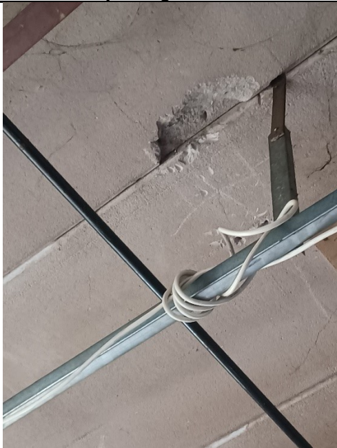
Damaged to RAAC plank
