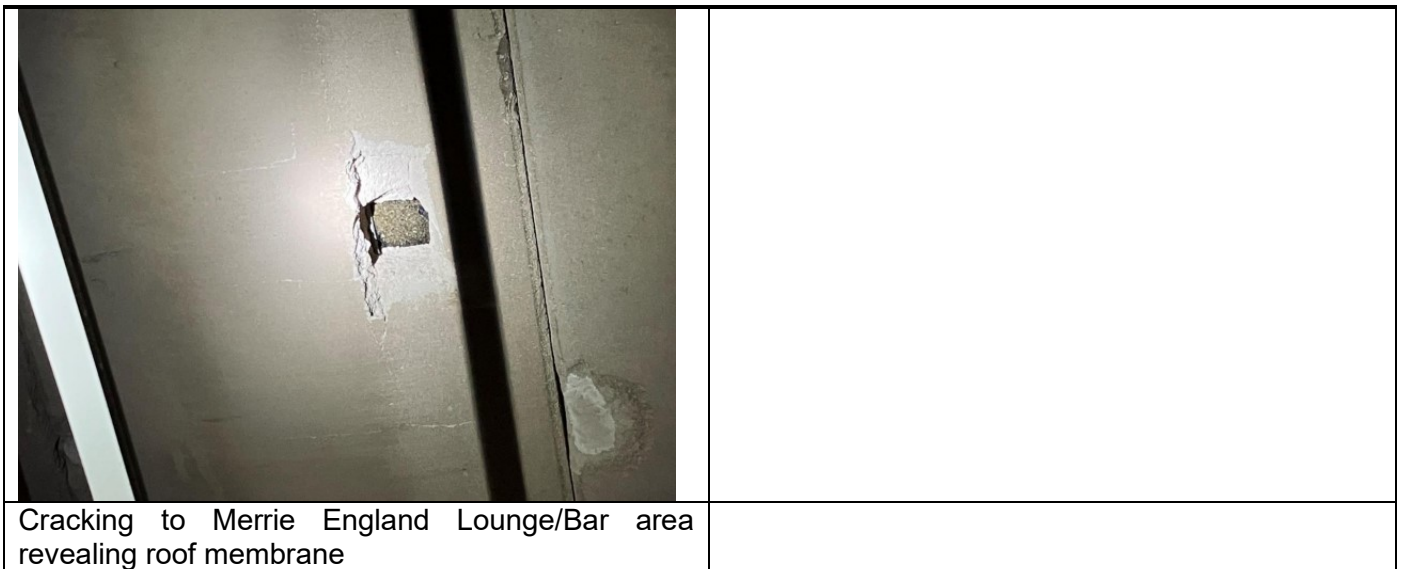
Figure 19 – Evidence of moisture ingress and roof exposure. Source Thomas Consulting (2023)
