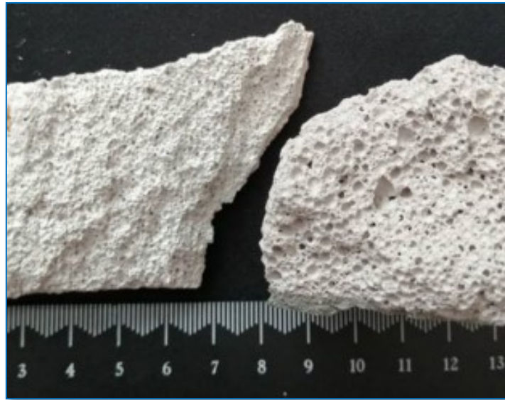
Figure 1 - Sample of texture of RAAC. Source Institution of Structural Engineers (2019)
