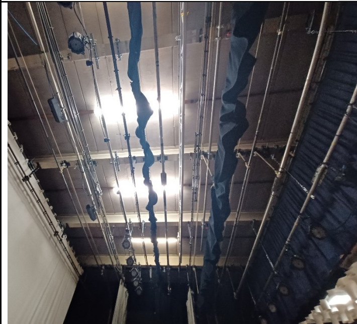
Theatre Stage area ceiling showing RAAC planks
