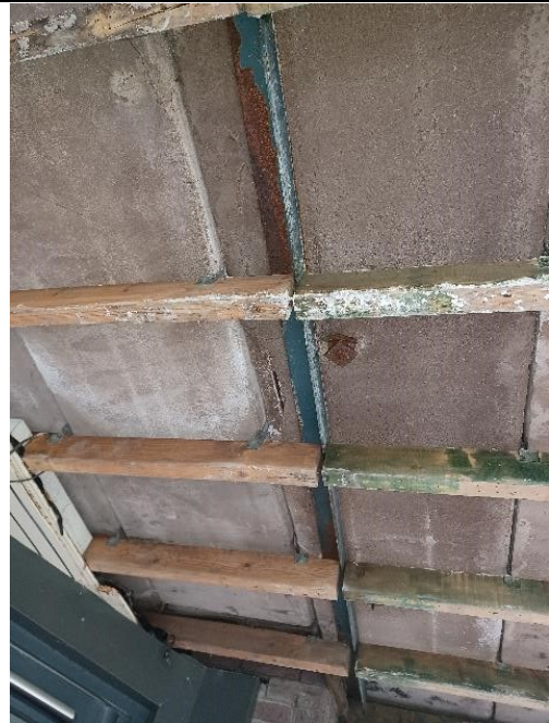
Covered internal walkway RAAC plank penetration, timber beam support and corrosion to steel work beam. Evidence of moisture ingress.
